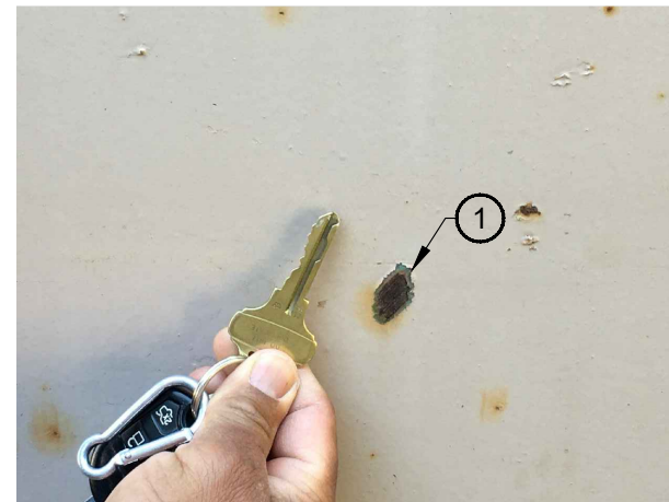
B RUST SPOT ON TANK WALL
