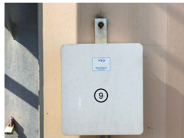
H CATHODIC PROTECTION PANEL
